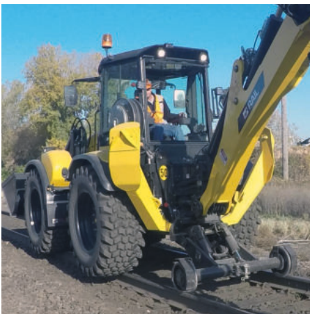
ABOVE: The Huddig Rail can get on and off railway tracks at any location, making work much more efficient
